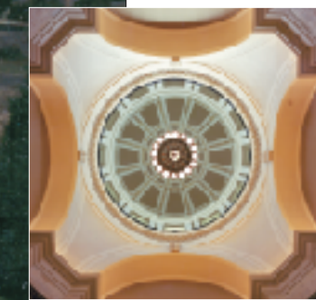
Below: Interior rotunda dome with its brass chandelier is the Capitol's grand focal point.
